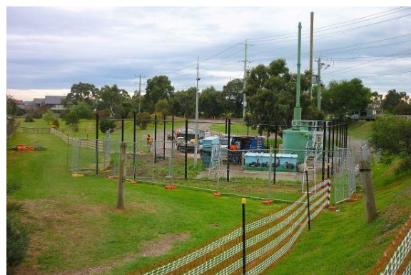
Figure 8: Sewer pumpstation with new perimeter fence
